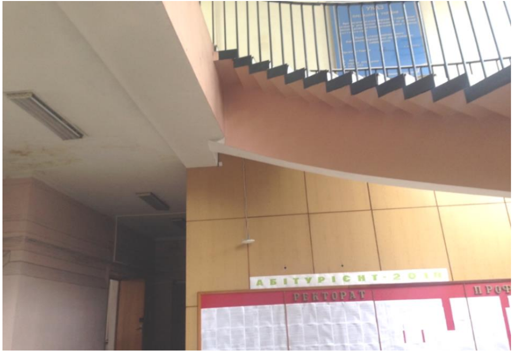
Fig. 3.45. Support of the curvilinear stair stringer beam on the monolithic reinforced concrete longitudinal floor beam of the second floor along axis "B", between axes "2-3", at elevation +3.900
