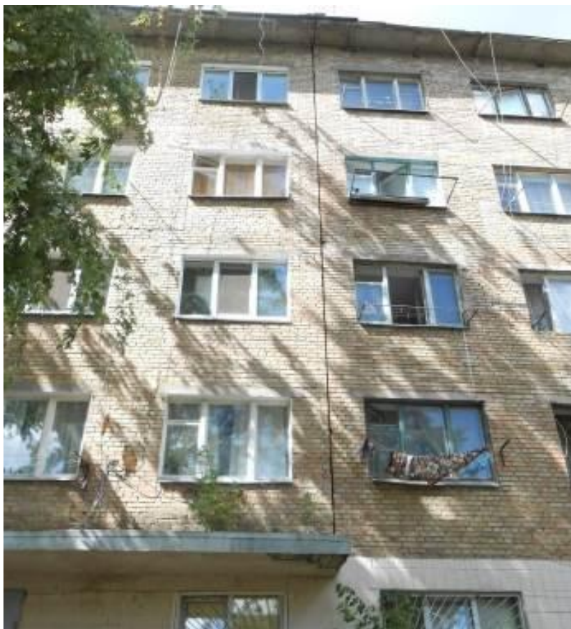
Fig. 3.20. Thermal expansion joint of the residential building along axis "5" between axes "A–H"
