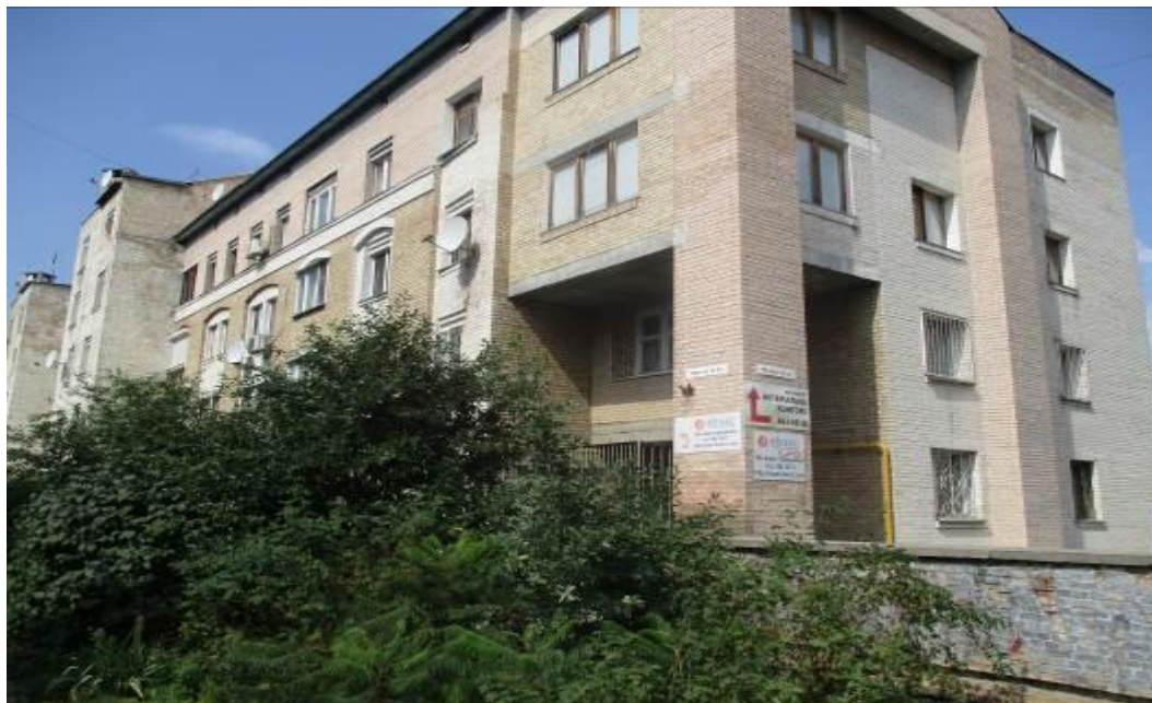
Fig. 3.15. Fragment of the building facade on Kyrylivska Street between axes "B–D" and "17–25"
