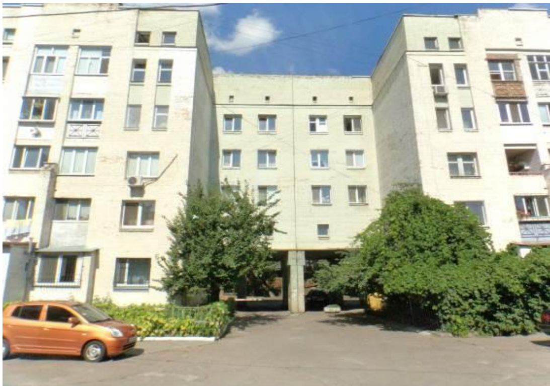
Fig. 3.11. Fragment of the courtyard facade of the building between axes "13–11", expansion joint.
