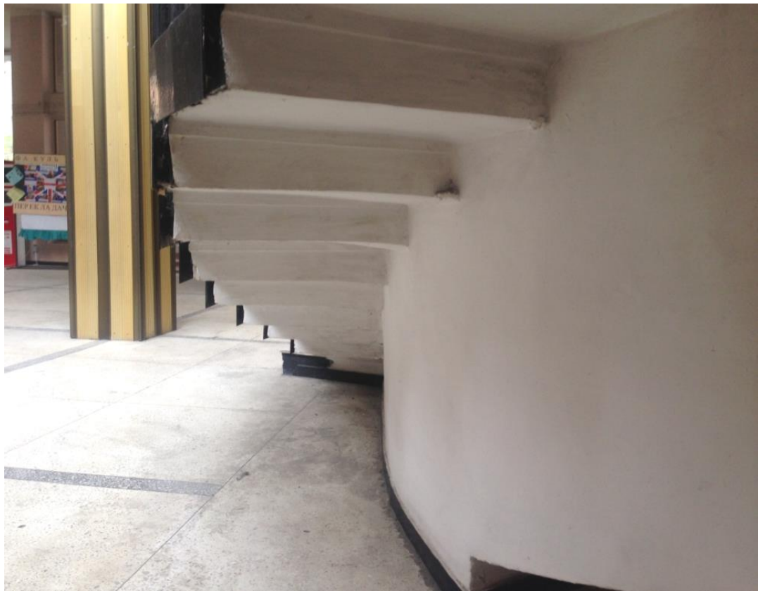
Fig. 3.46. Support of monolithic reinforced concrete trapezoidal steps on the curvilinear beam between axes "2-4", "B-H", at elevation -1.100...0.000
