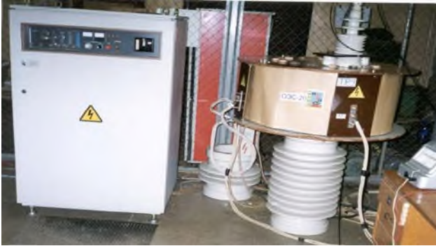
Fig. 7. 20 kW, 1 kHz resonant electric power transmission system.
