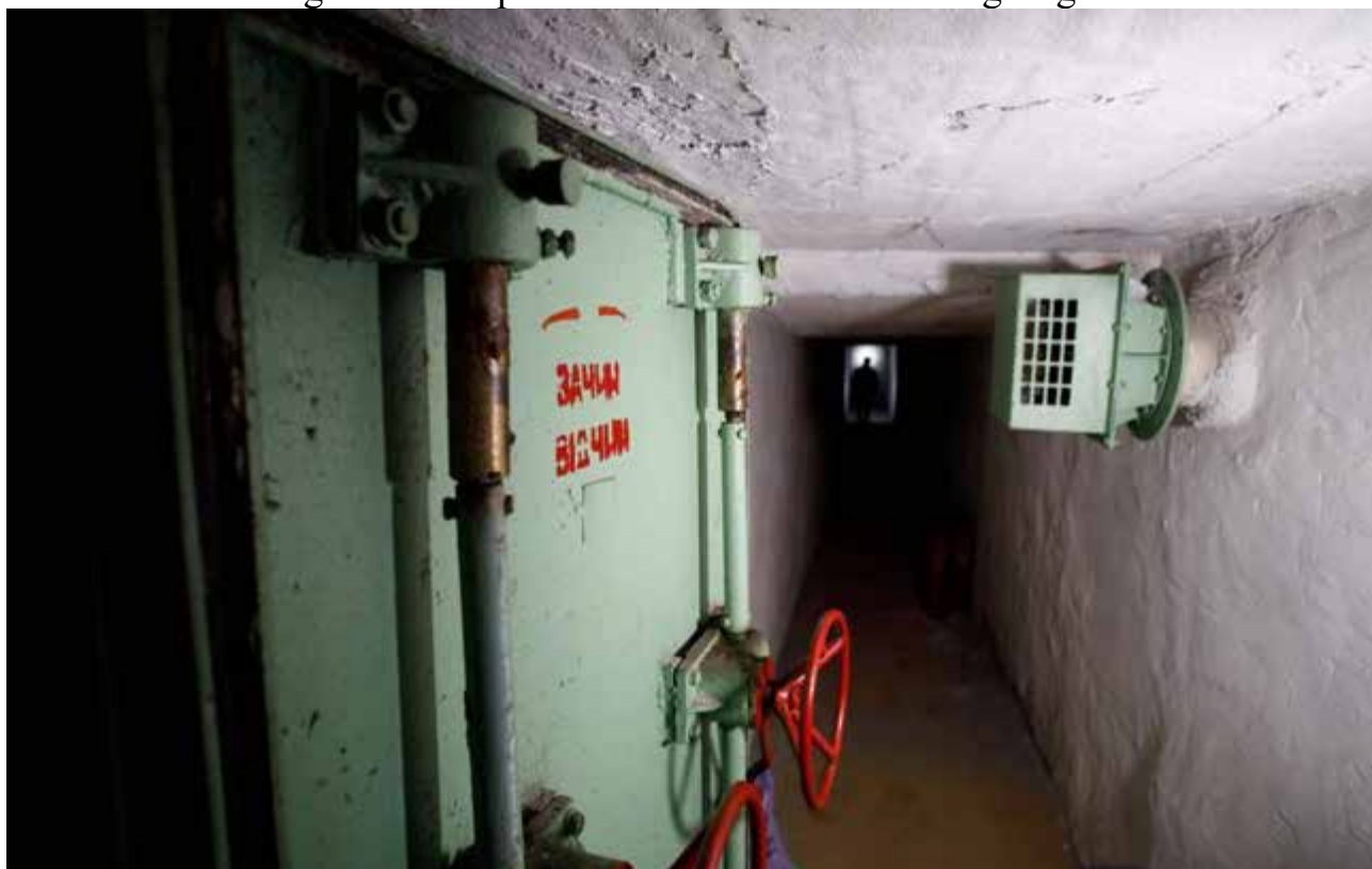
Photo 1. Bomb shelters must have two exits and ventilation
