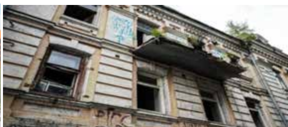
Fig. 2 A building that needs renovation
