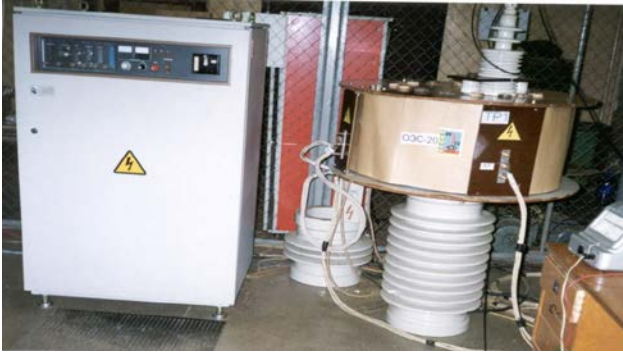
Fig. 7. 20 kW, 1 kHz resonant electric power transmission system.
